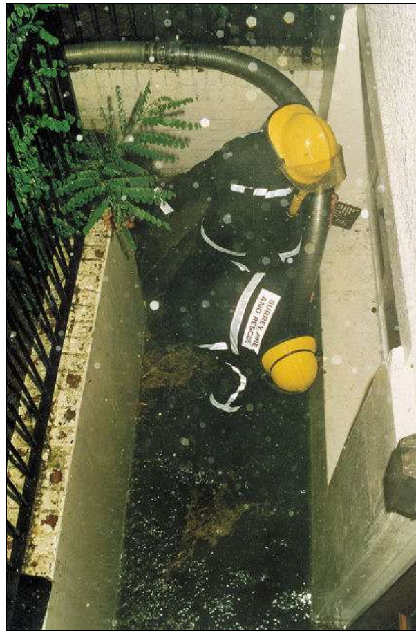
Men from Surrey Fire and Rescue pumping out a flooded basement in Temple Road. Date Not Known
